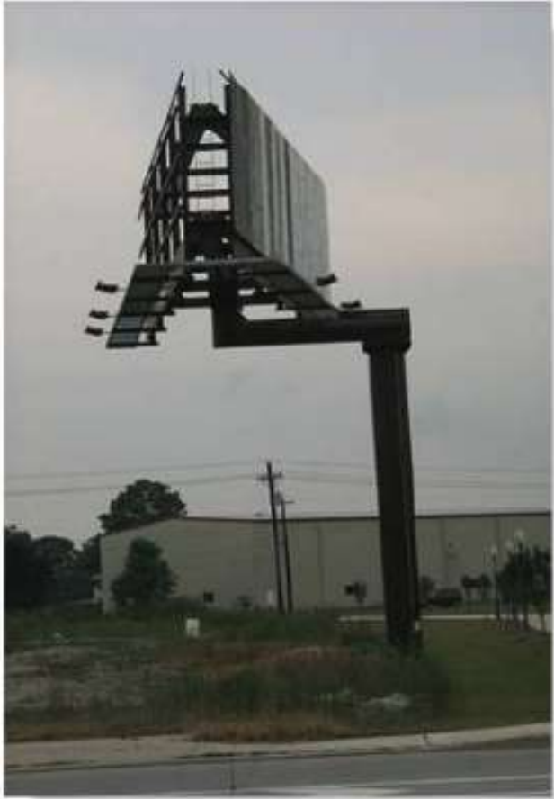
The weight of this sign and the wind loadings acting on it will cause normal and shear forces and bending and torsional moments in the supporting column.
